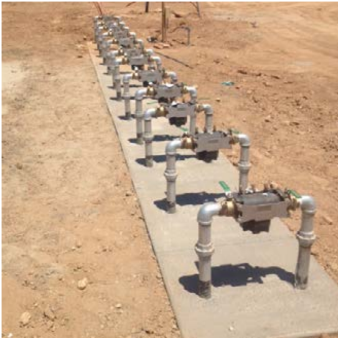
375XL Reduced Pressure Principle Assemblies installed in a commercial shopping center
